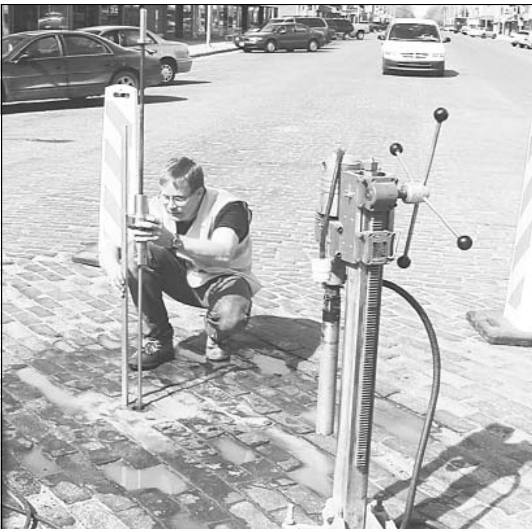
Jerry Nemecheck, an engineer with Evans, Bierly, Hutchison Associates, drilled holes in the intersections at 11th and 12th and Main on Friday as the first step in replacing the old bricks. He said the tests were to determine the condition of the base under the bricks so the firm can design the new intersections to be done this year. Photo by Tom Betz / The Goodland Star-News
