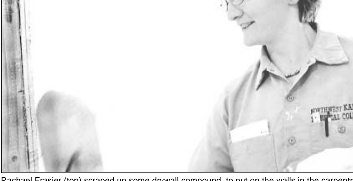
Rachael Frasier (top) scraped up some drywall compound to put on the walls in the carpentry department's project house. Emily Pelster (above) smoothed some compound onto another wall in the house.
