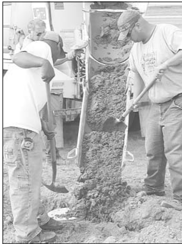
Ronald Edmond (left) and Jason Yartz, both of Girard, spread cement around one of the cans that will be used as a base for the lights being installed on the crosswind runway at Renner Field. Strukel Electric of Girard won the contract for the project, for which about 80 percent is being paid by a state grant.
