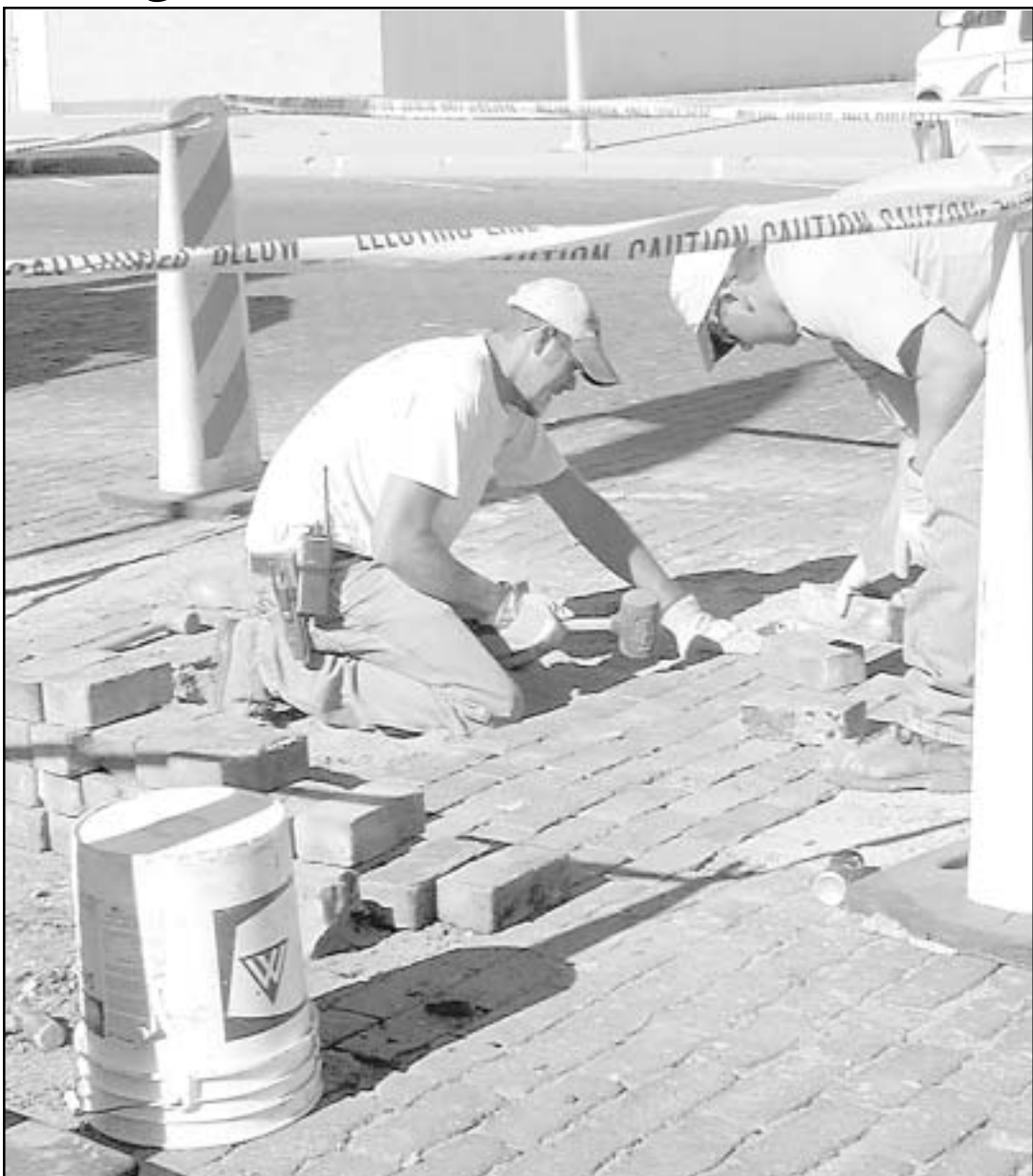
City worker Joey Snethen hammered bricks on Main Ave. on Friday, July 29, after a water leak forced the crew to tear up the street in front of American Communications.
