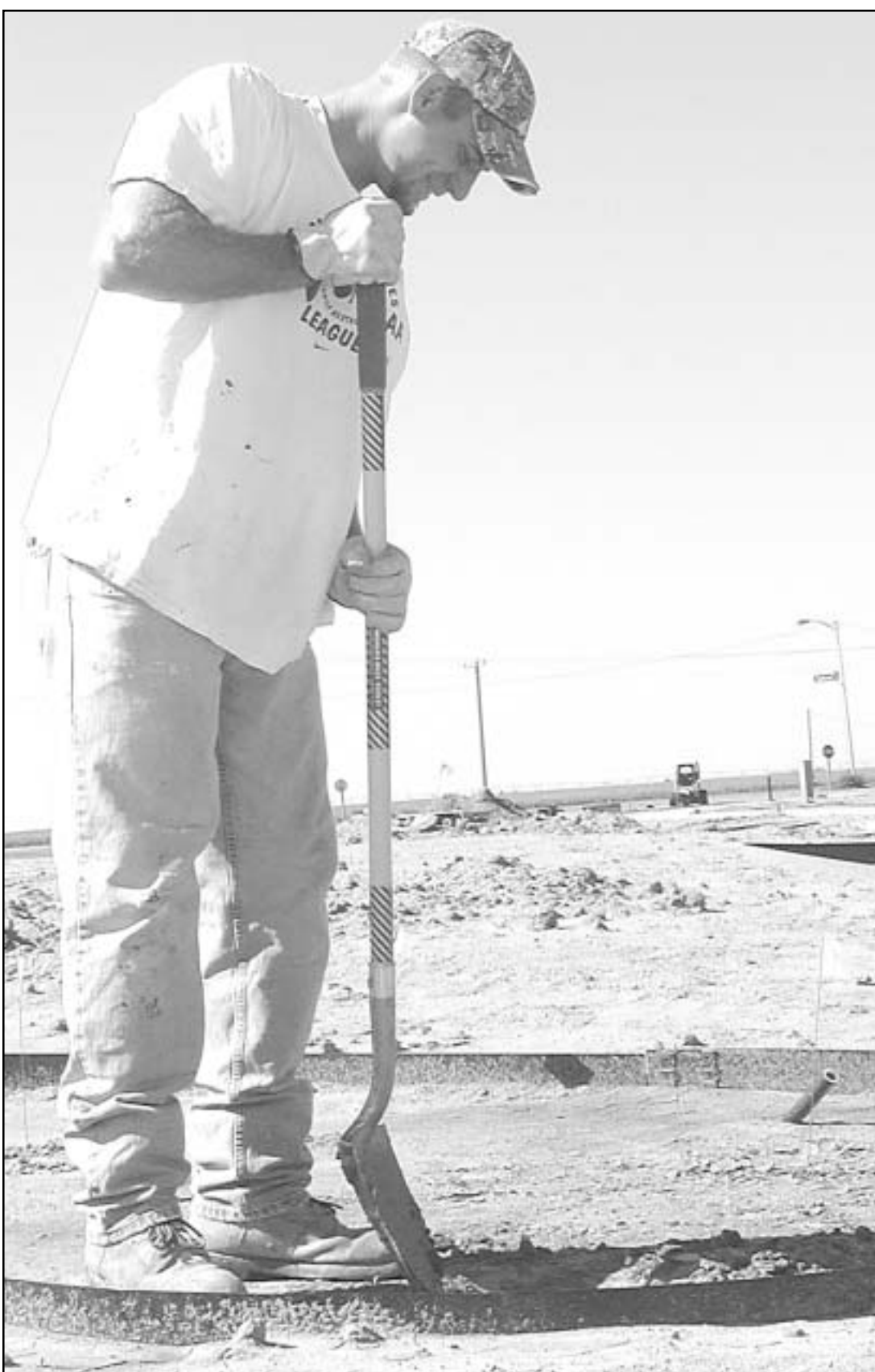
Mike Bohme with Miller Construction helped the crew dig holes for plants at Pioneer Park last week. The park is starting to take shape as the contractor moves toward an October completion date.
