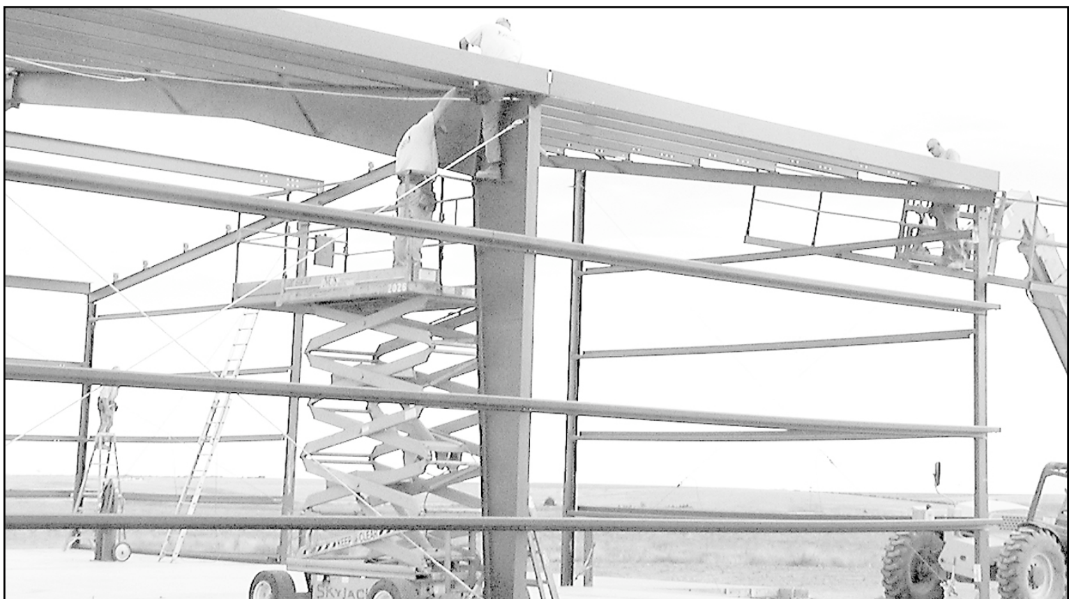
Mark Van Patten, (sitting on top), worked with Travis Hogan to line up holes for an I-beam of the warehouse at the Goodland Energy
