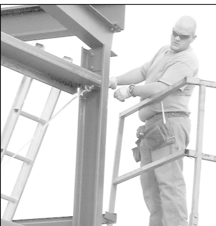
Matt Van Patten of Northwest Central Kansas checked the alignment of an I-beam on the warehouse being erected at the Goodland Energy Center. Photo by Tom Betz/The Goodland Star-News
