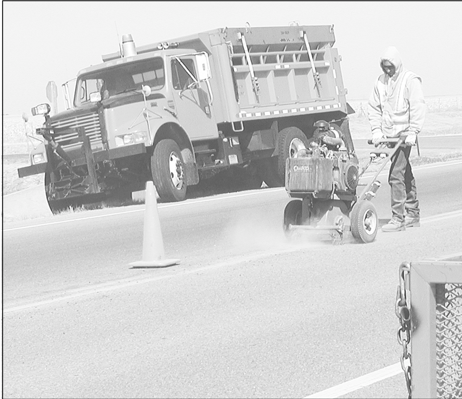
Kansas Department of Transportation workers were out in the wind Friday, working on the pavement on K-27 by Eighth Street. Warmer weather signals the beginning of road work. Photo by Pat Schiefen/The Goodland Star-News
