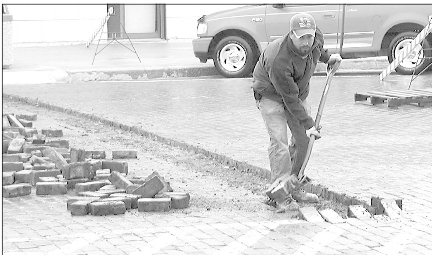
Miller Construction started removing bricks from the intersection of 10th and Main on Monday. It is first of the five intersections on Main Avenue the firm will rebuild this summer. Ben Ramirez was using a shovel to pry up bricks. The Goodland
