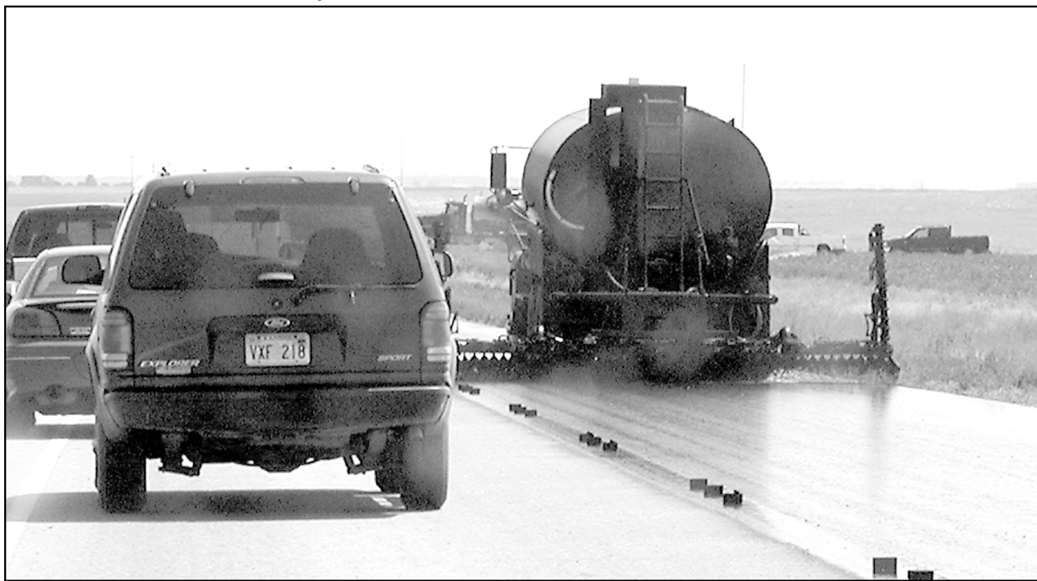
There was one-lane traffic on K-27 north of Goodland on Tuesday as Hi-Plains Sand of Kanopolis chip sealed the 16.5 miles of highway from Business U.S. 24 to the Cheyenne County line. Eric Oelschlager, area engineer from Atwood, said the project, cost of $333,000, is designed to protect the new asphalt surface. Photo by Tom Betz/The Goodland Star-News
