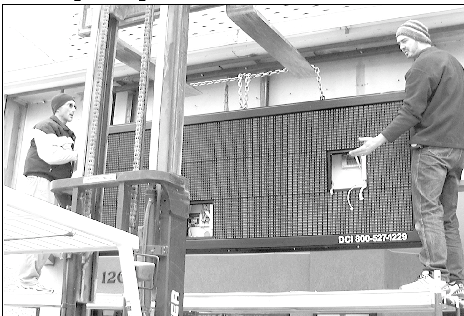
The weather turned cold Wednesday, but a crew hoisted a new digital marquee for the Sherman Theatre into place and hooked it up. Owner Dave Branda (left) held on to one side while Brian Freeman of the Goodland Grind and Gallery held the other and
