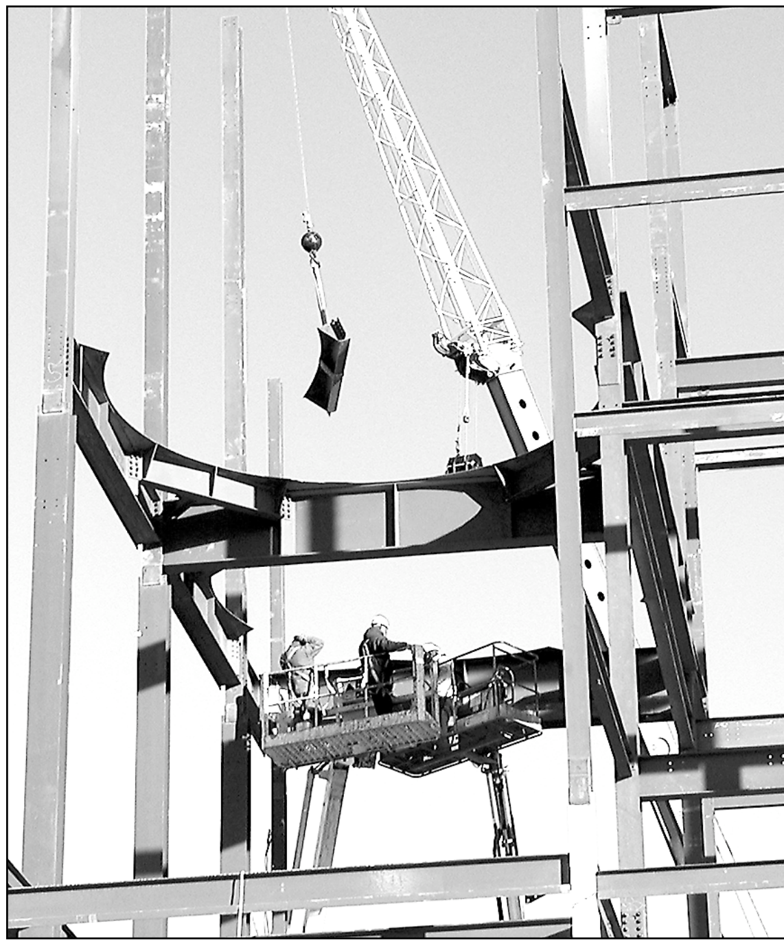
A section of the collar for the coal bunker for the Goodland Energy Resources power plant was lifted into place at the site north of Caruso as Goodland High School students watched.
