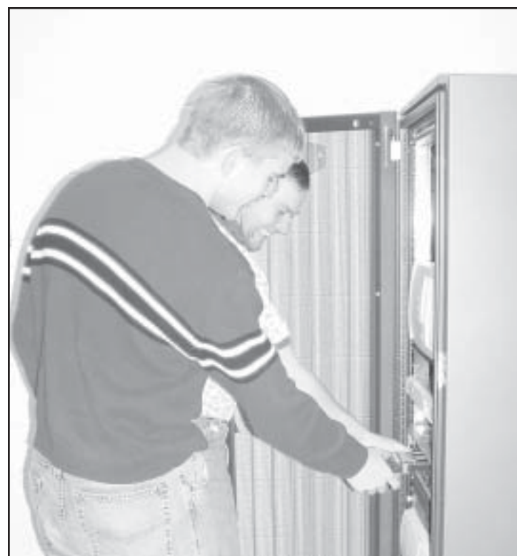
CHECKING OUT THE EQUIPMENT , Jake Robinson (front) and Jess Randel were working to get everything ready to webcast the Oberlin Invitational. —Herald staff photo
