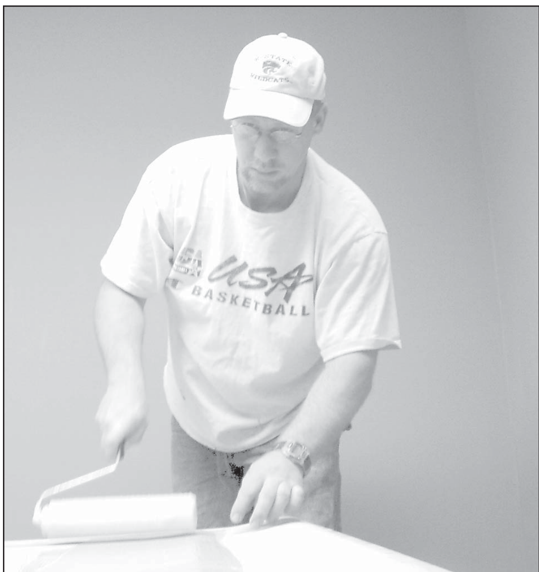
WITH ROLLER IN HAND , an employee from Schultz's of St. Francis, was busy wallpapering the vault at First National Bank as part of the renovation project.
