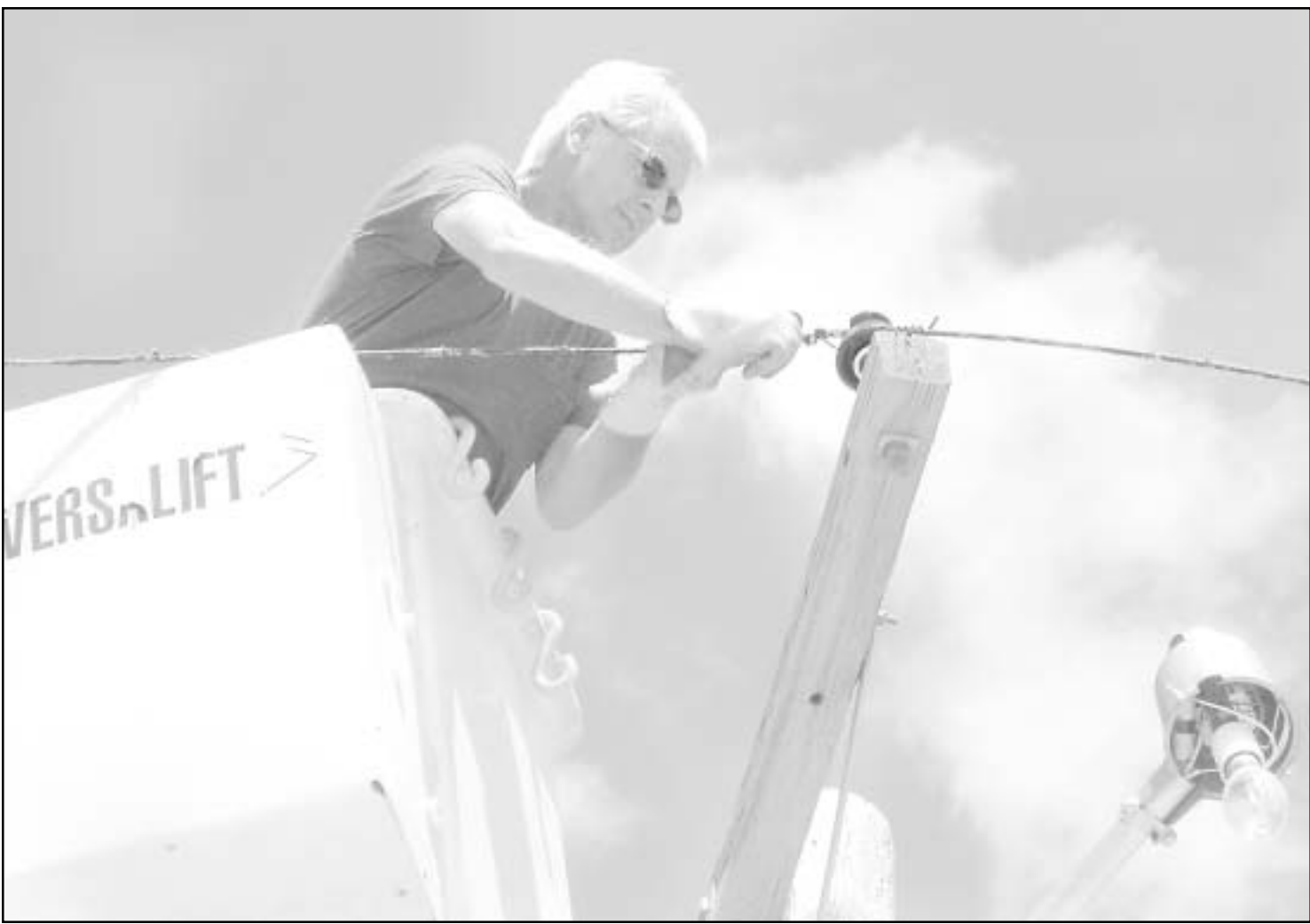
FRIDAY AFTERNOON , Ron Beneda worked from a bucket truck to prepare power lines behind the high school for a pole replacement after an employee of J Corp, the company doing the city water project, hit the pole with a back hoe. The broken pole is on the south side of high school parking lot. — Herald staff photo by Kimberly Brandt
