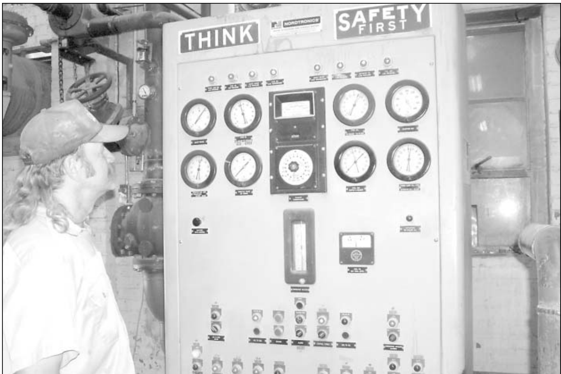
JUST TO MAKE SURE everything ran smoothly, Foreman Dan Castle checked the gages of an engine at the city power plant. —Staff photo by Kimberly Brandt
