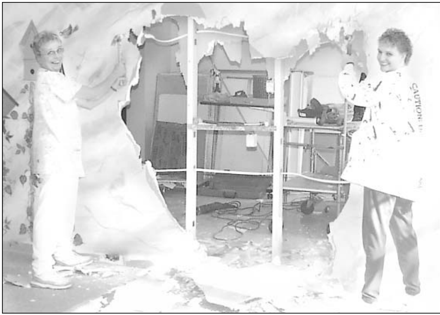
HAMMERS IN HAND , nurse Becky Alstrom (left) and unit coordinator JuliAnna Baker helped tear down a wall to make a new, more home-like eating area for the Angel Lane neighborhood at the Good Samaritan Center.
