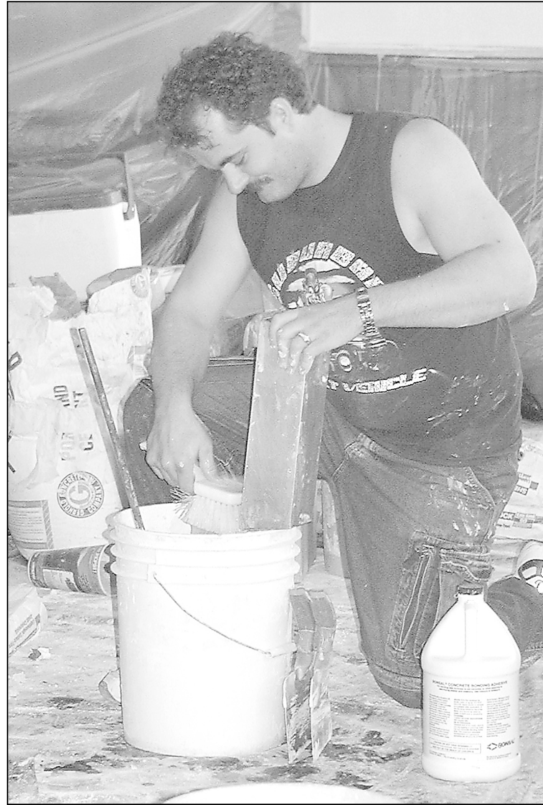
A WORKER FROM Roger Goltl's drywall business in McCook was finishing the walls in the old Bohemian Hall last week. — Herald staff photo by Kimberly Brandt
