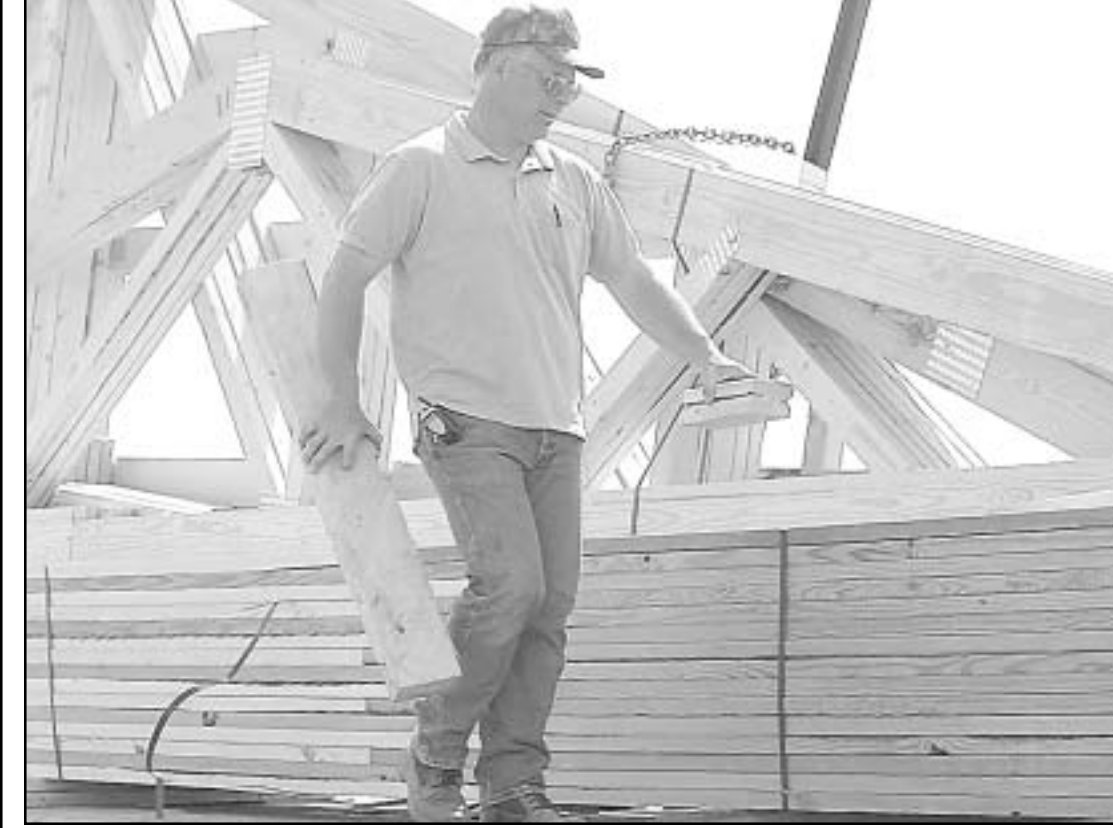
WITH WOOD IN HIS HANDS , Kevin Brown, owner of Sappa Valley Construction, helped unload materials to build a new shop and office for his business on U.S. 83 just north of town.
