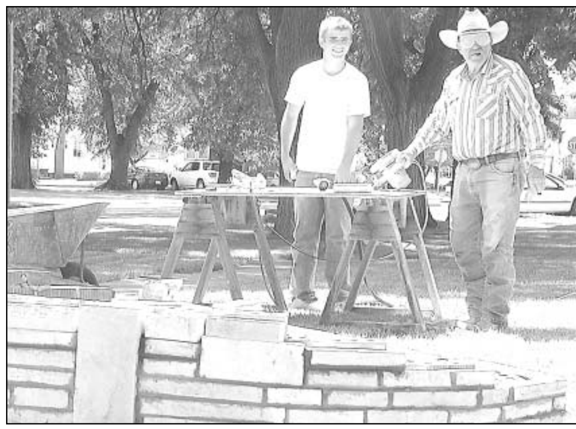
PUTTING UP A ROCK PLANTER in the front yard, Jerry Lohofener cut and fitted natural stone around a brick base last week with the help of his grandson, Jace Robinson.
