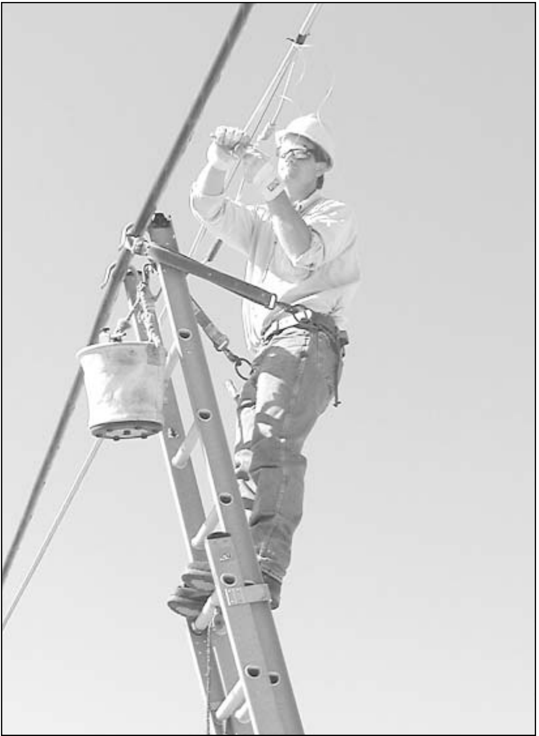
WITH A BELT AROUND HIS WAIST and his feet placed firmly on a ladder, Mike Kolar, with Cebridge Connections, fixed a break in the cable 12 to 15 feet above Dave Nichols' house on U.S. 36 last Wednesday. — Herald staff photo by Cynthia Haynes
