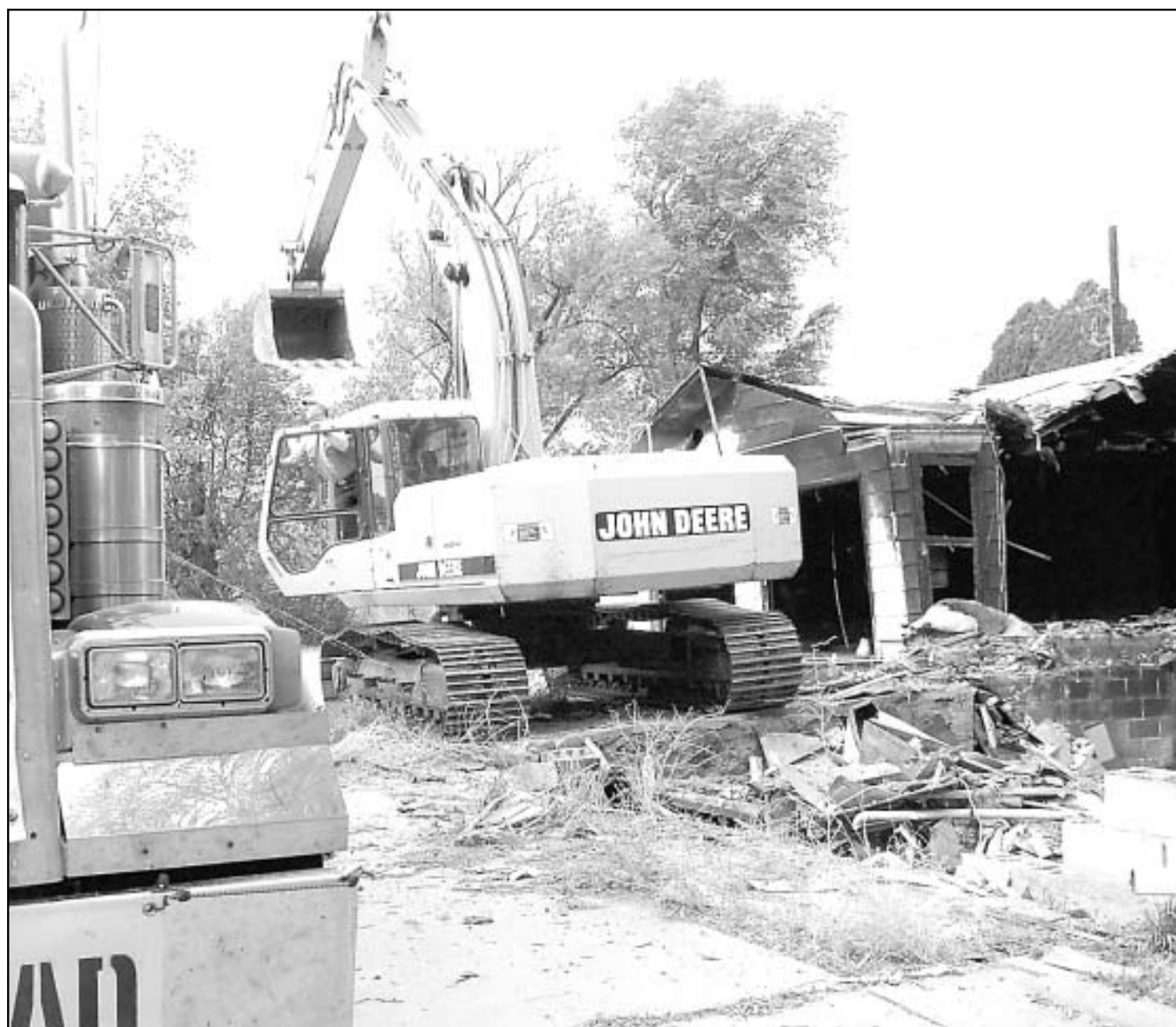
AFTER LUNCH Friday, Douglas Cass with Cass Excavating of Hoxie, used a loader to tear down Edna Mott's house, which was damaged by fire last May. — Herald staff photo by Karla Jones
