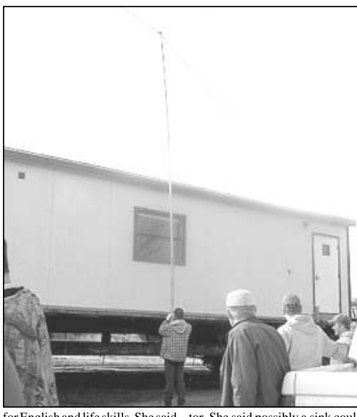
for English and life skills. She said she would like a 220 electric line added so an electric range could be put in and a 110 line for a refrigerator.
