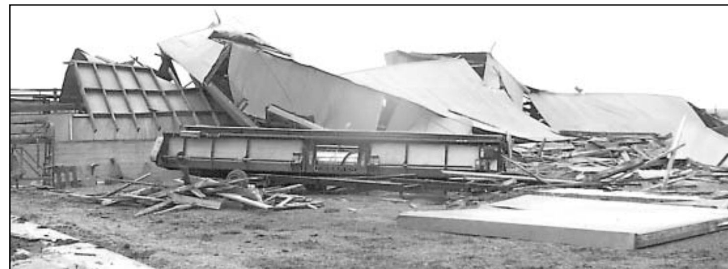
THE COW PALACE , a cattle barn which has been a landmark for many years 15 miles south of Oberlin on U.S. 83, fell last month when high winds or a twister came through around 7 p.m. Owner Brad Marcuson said they were washing 4-H calves at their home about that time and noticed that
