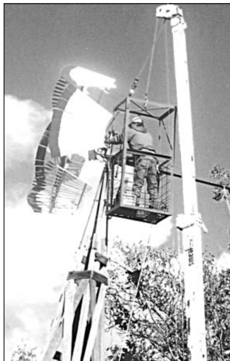
A TALL CRANE carefully lifted the restored windmill head onto a wooden tower at the Cottonwood Ranch near Studley.
