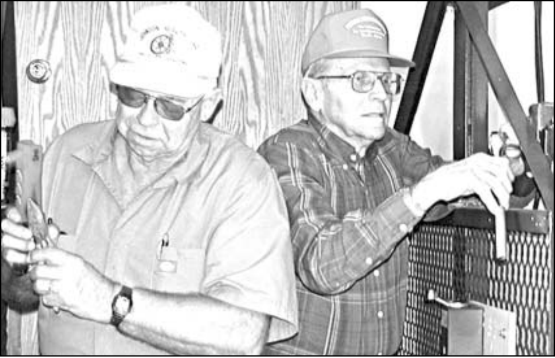
WORKING TOGETHER , volunteers Don Fredrickson (left) and Lawrence Wenger made the finishing touches for a new elevator at the United Church of Oberlin. The elevator was donated by Mr. Wenger and his children, Judy Wenger of Oberlin and Norbert Wenger of Yukon, Okla., in memory of Cleta Wenger. Money for other expenses came from funds given in memory of Howard Banta, Loretta Nelson and Gustave Lippelmann.
