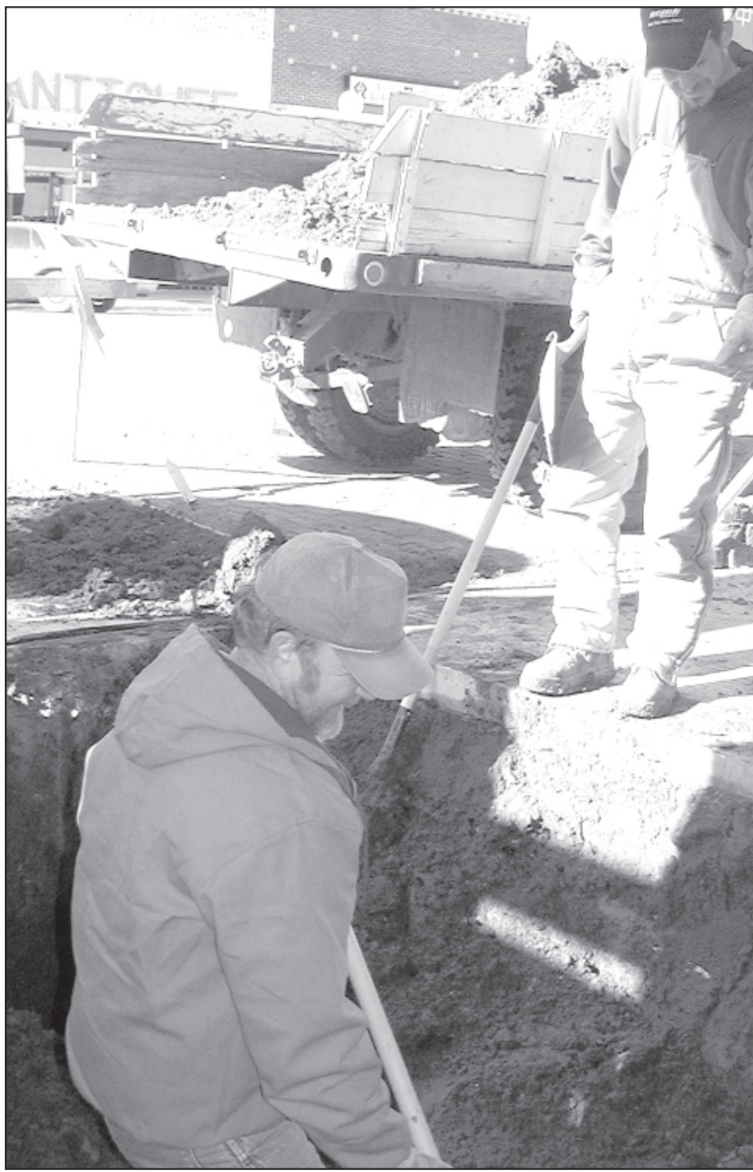
ON MAIN STREET LAST MONDAY , David Sporn, with the city water department, and city Foreman Dan Castle (above) worked to get a larger water pipe under the sidewalk to go into the new coin laundry.
