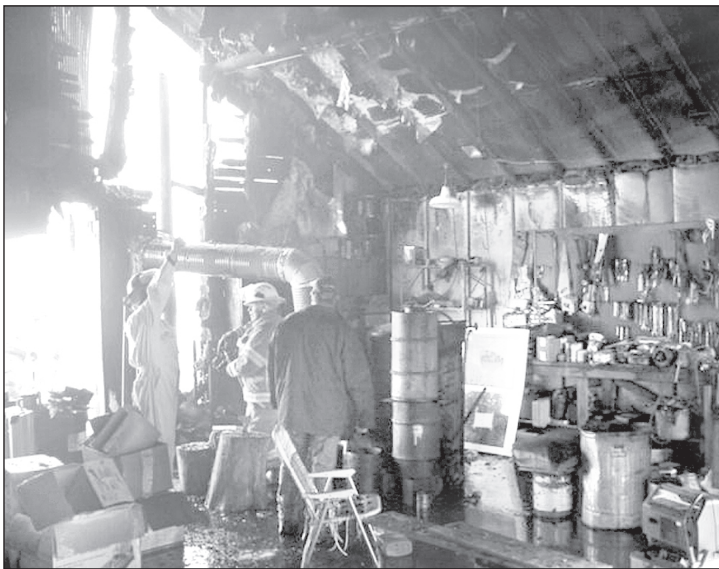
DECATUR COUNTY FIREFIGHTERS put out flames in Millard Kyte's shop last Tuesday after a leak in the chimney of a wood-burning stove started a fire. Damage was heavy inside the shop. — Photo by Randy McHugh
