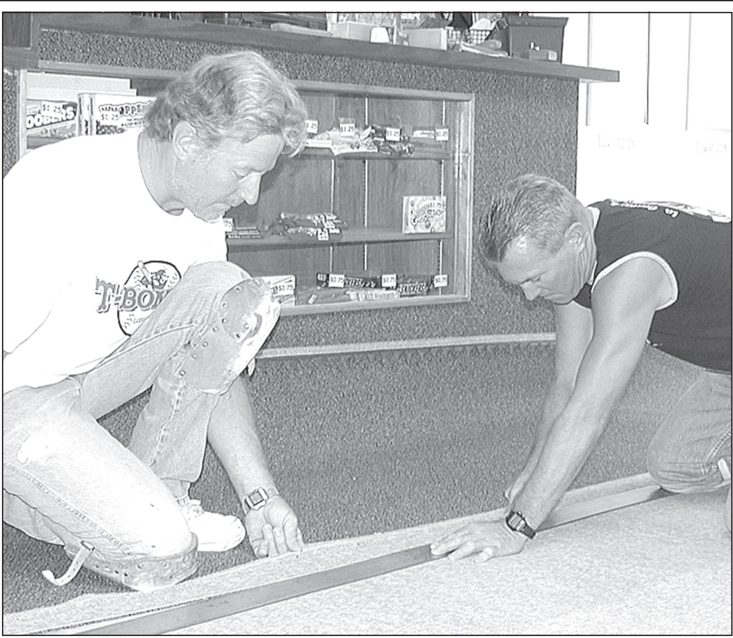
AT SUNFLOWER CINEMA, brothers Steve (left) and Ron Diederich volunteered their time and supplies to install new carpet purchased from the Carpet Center with money raised by the board. — Herald staff photo by Kimberly Davis
