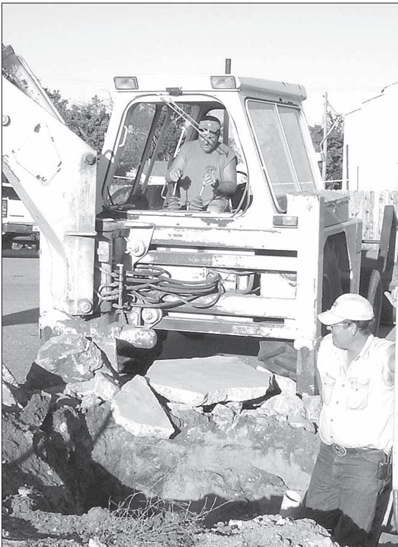
IN THE BACKHOE, Leroy Spresser dug down to the water line with the assistance of Greg Bruggeman.
