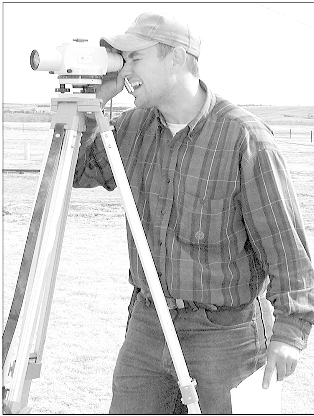
ON SATURDAY Michael Wasson used survey equipment at the Decatur County Fairground to start the leveling work for the new arena and livestock building purchased through the Decatur County Fair Foundation. Mr. Wasson and Clay Anderson, who also helped with the leveling, spearheaded the fundraising for the building.
