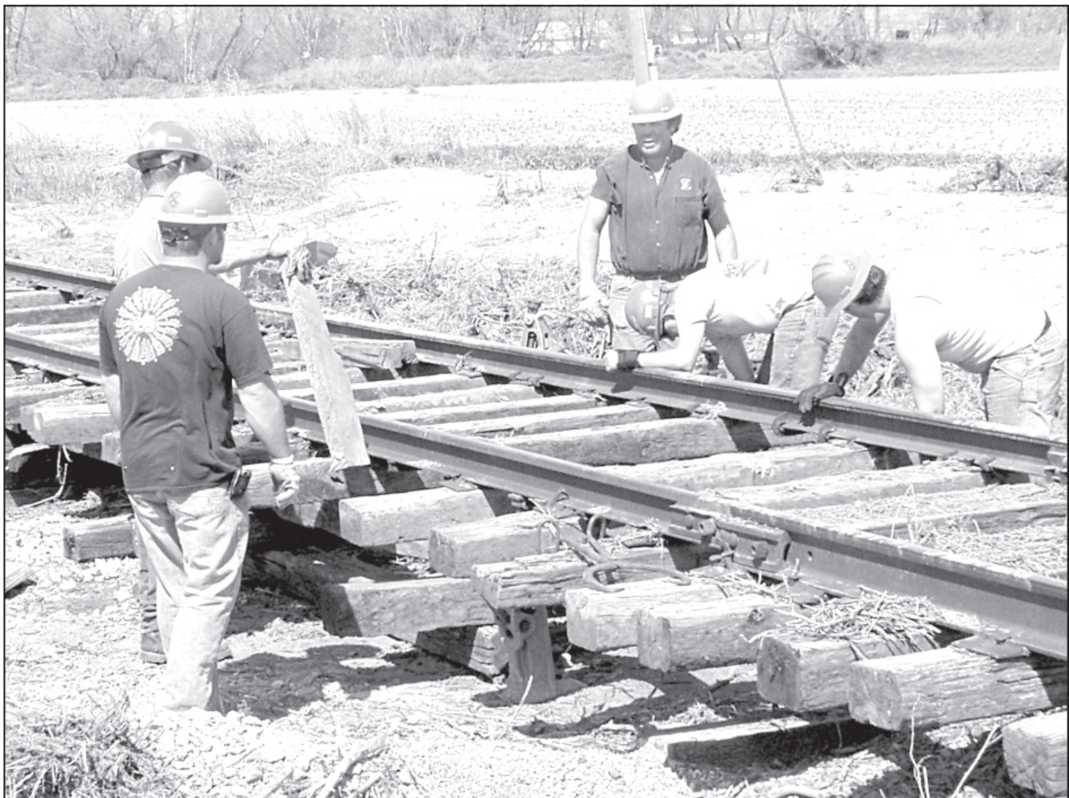
OUTSIDE OF HERNDON, a Nebraska-Kansas-Colorado RailNet crew worked Monday morning to fix the track washed
