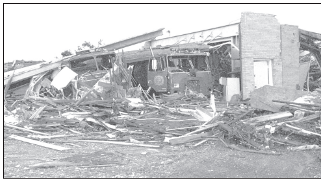
THE ROOF on the fire station in Greensburg fell in during a tornado at the beginning of the month. — Photo by Steve Hirsch
