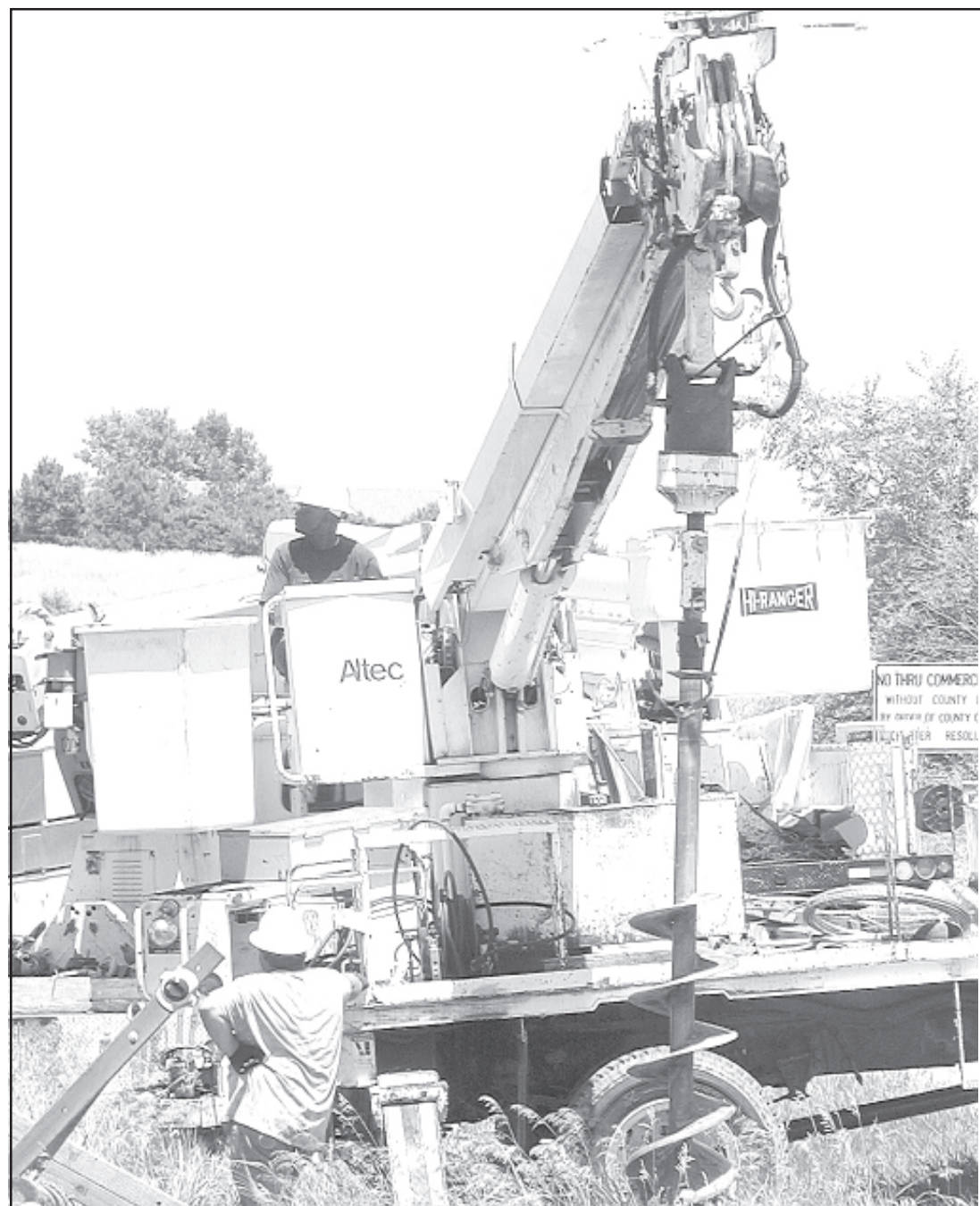
ACROSS FROM the Oberlin Cemetery, a crew from C&H Powerline replaced a pole on a Prairie Land Electric line last week. The company is rebuilding lines throughout the area for the cooperative.
