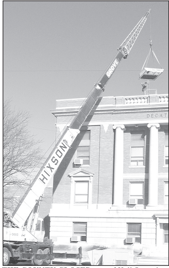
THE COUNTY CLOSED part of Hall Street last Tuesday while a large crane and crew of men put a new heater and air conditioner on the roof of the courthouse
