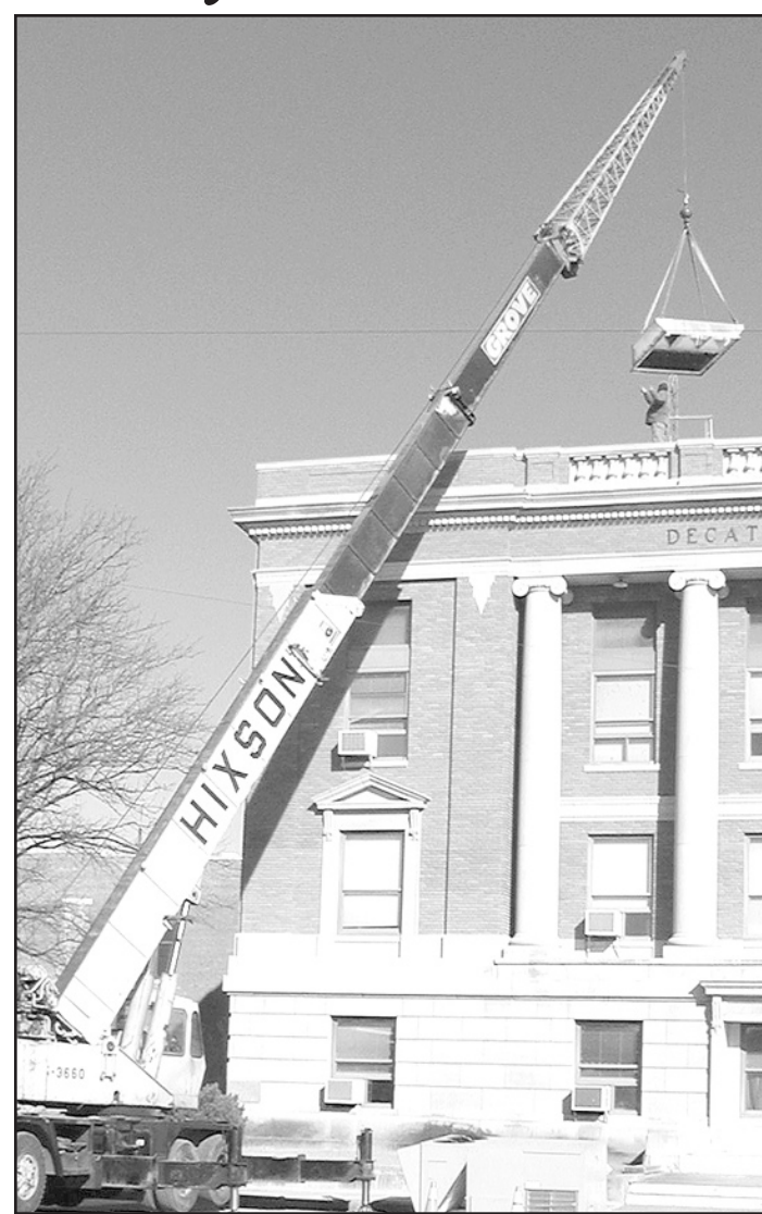
THE COUNTY CLOSED part of Hall Street last Tuesday while a large crane and crew of men put a new heater and air conditioner on the roof of the courthouse — Herald staff photo by Kimberly Davis.
