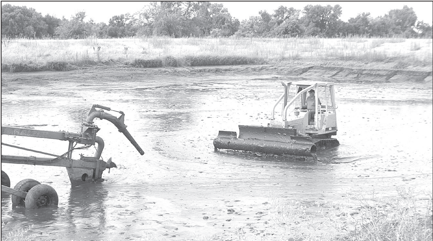
AT THE CITY'S OLD waste water treatment plant, a worker holding pond while (below) another spread the sludge (above) with Liquid Waste Management cleaned out the old on a nearby city-owned field.
