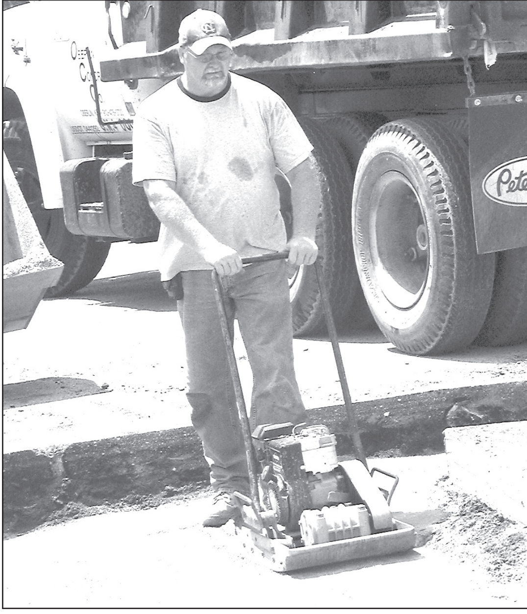
ON WEST HALL STREET near Elk Avenue on Monday, Glen Stragey with Oberlin Concrete prepared dirt to replace part of the street near the corner. City Administrator Gary Shike said the city wants to put in a curb and a new section of pavement for drainage.
