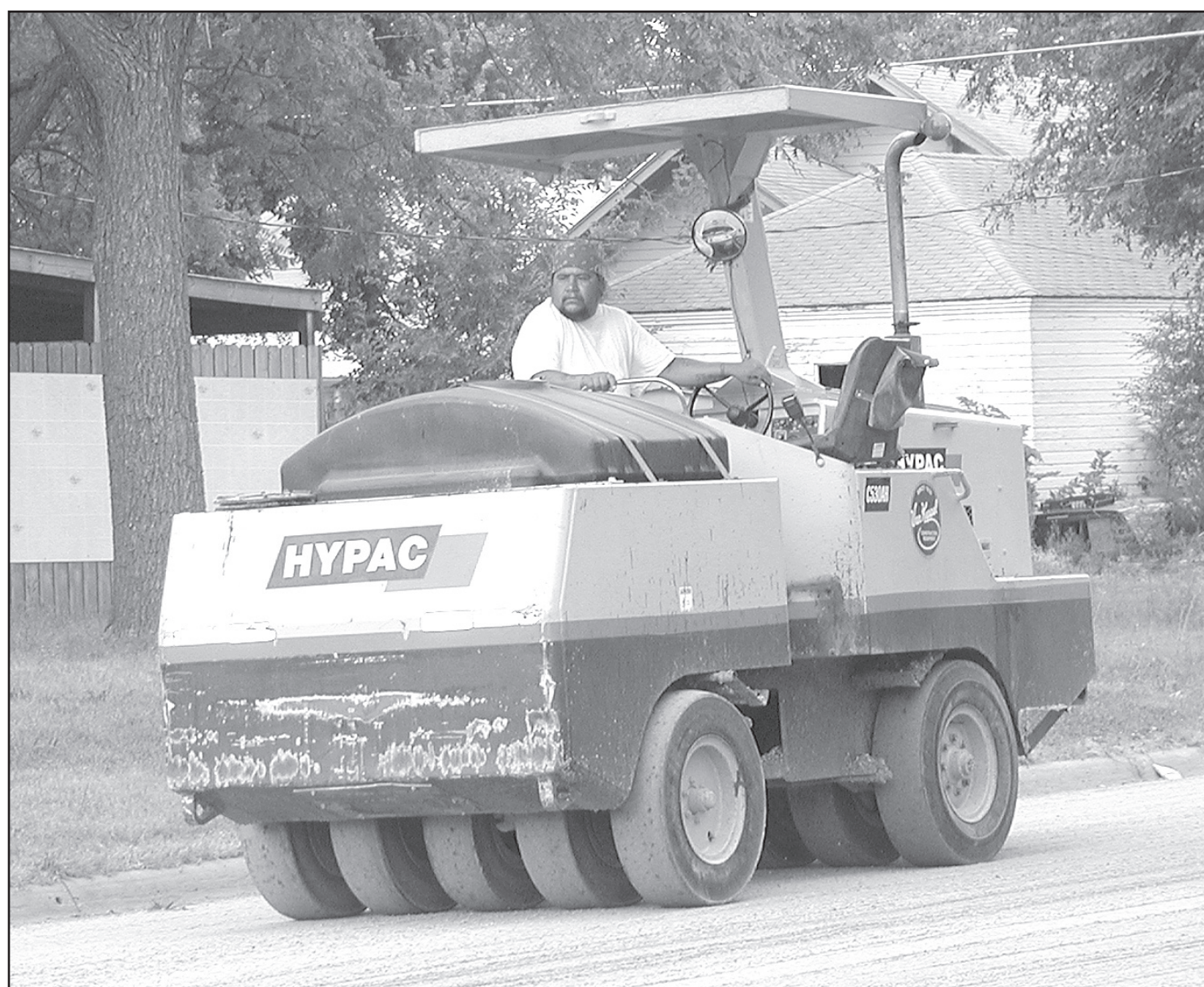
ON MAPLE STREET Monday morning, an employee of B&H Paving out of Scott City drove a machine to pack the sand during the street sealing process. — Herald staff photo by Kimberly Davis
