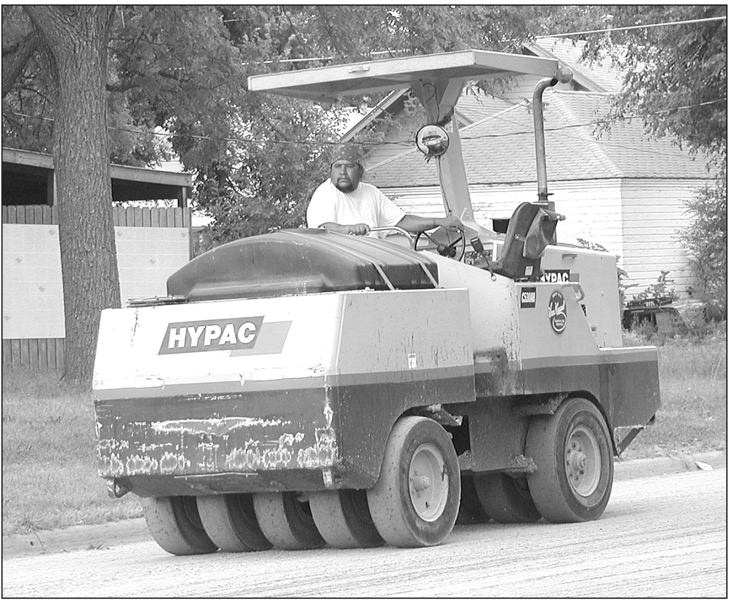
ON MAPLE STREET Monday morning, an employee of sand during the street sealing process. B&H Paving out of Scott City drove a machine to pack the — Herald staff photo by Kimberly Davis
