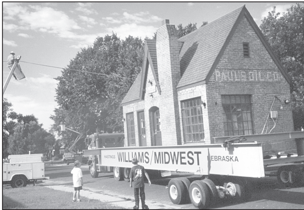
PAUL'S OIL COMPANY , originally located at the intersection of U.S. 36 and 83 highways, was moved to the museum by William/Midwest Movers of Hastings, Neb. It was originally owned by Paul Nitsch Sr.
