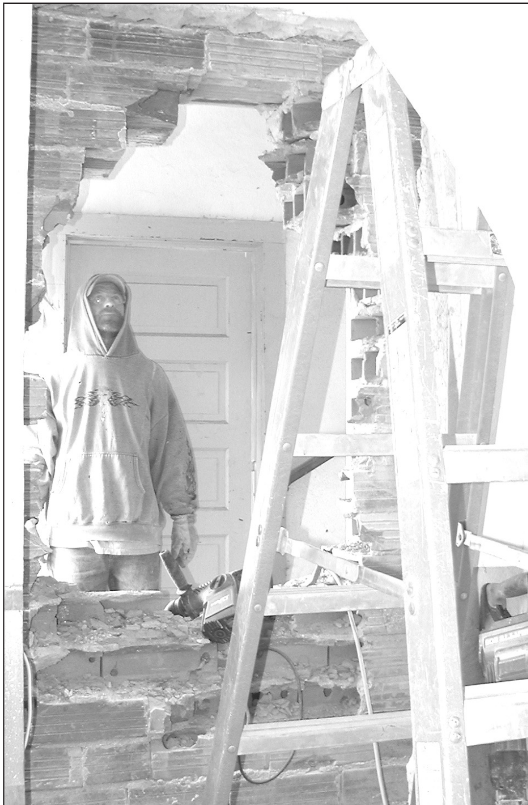
LAST WEDNESDAY, men with Doak Construction cut out a brick wall between the Last Indian Raid Museum's gift shop and the newly purchased building to the south, which will house the office.
