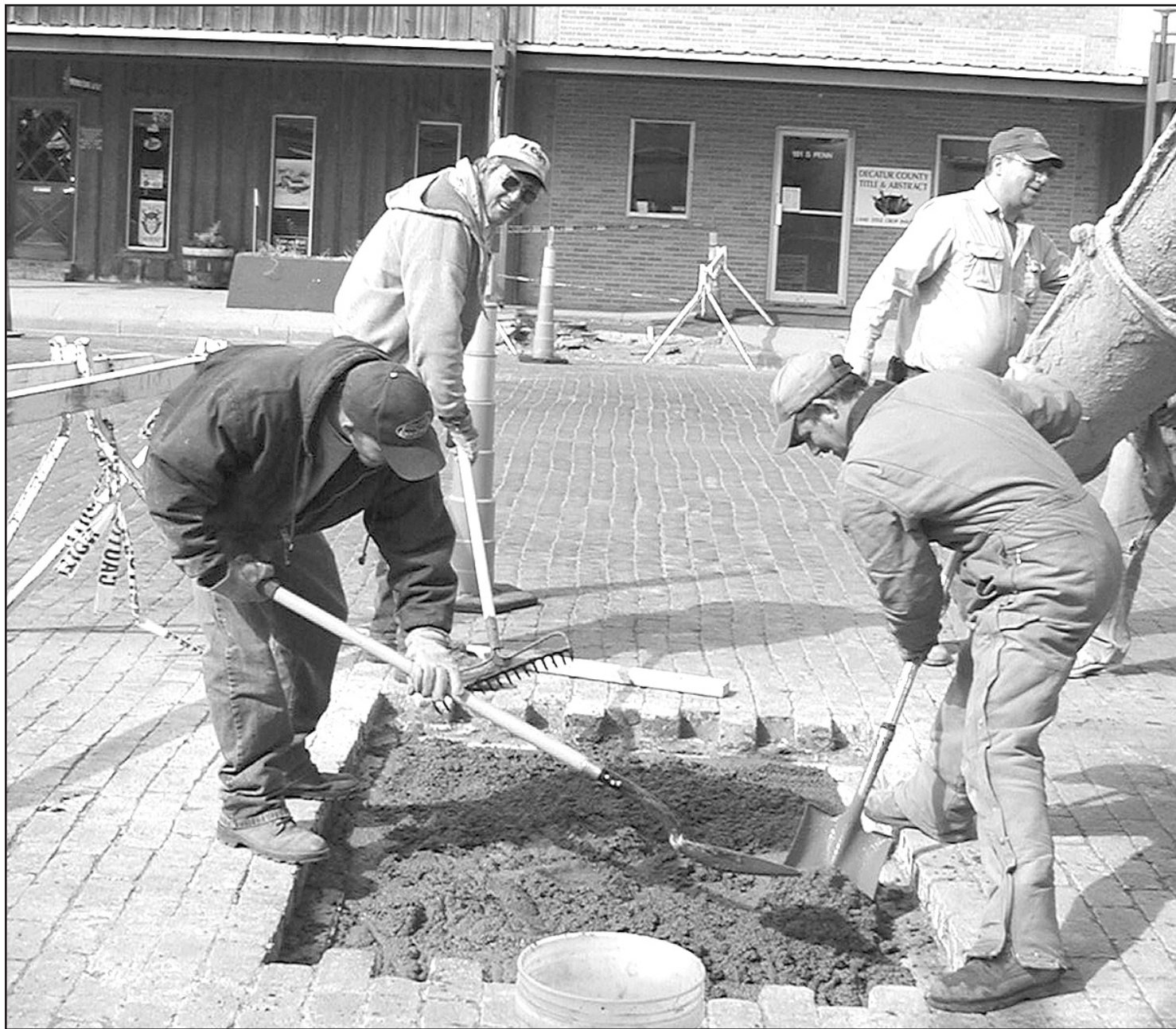
ON MAIN STREET last week Willard Perrin (back), Dan Dempewolf and David Sporn used a rake and shovels to level out concrete that covered a new water line the men had just replaced.
