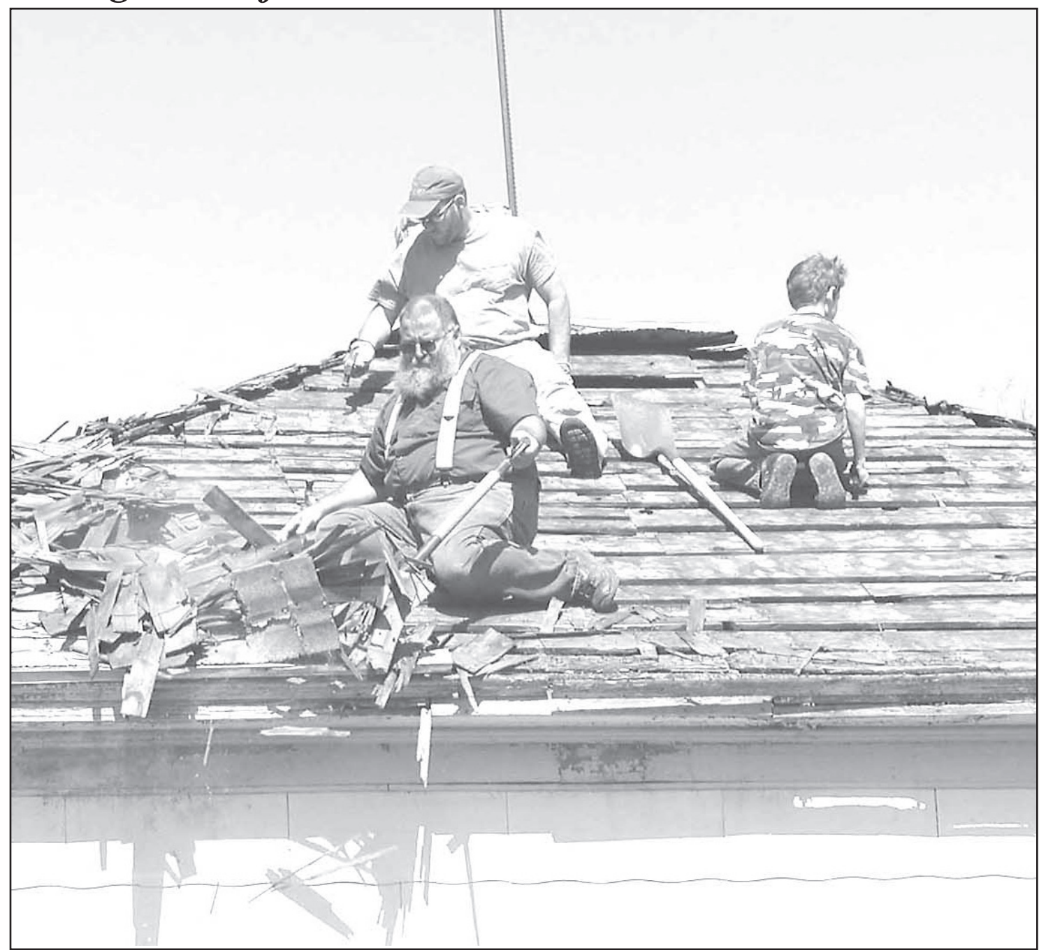
WITH THE SUN SHINING and temperatures in the high 70s, Rob McFee and his brother Tim and nephew Joe McFee of Atwood, worked to remove the old roofing from a small house at 313 W. Oak on Sunday. Rob owns the place, which he says he's fixing up to use for something, sometime. — Herald staff photo by Cynthia Haynes
