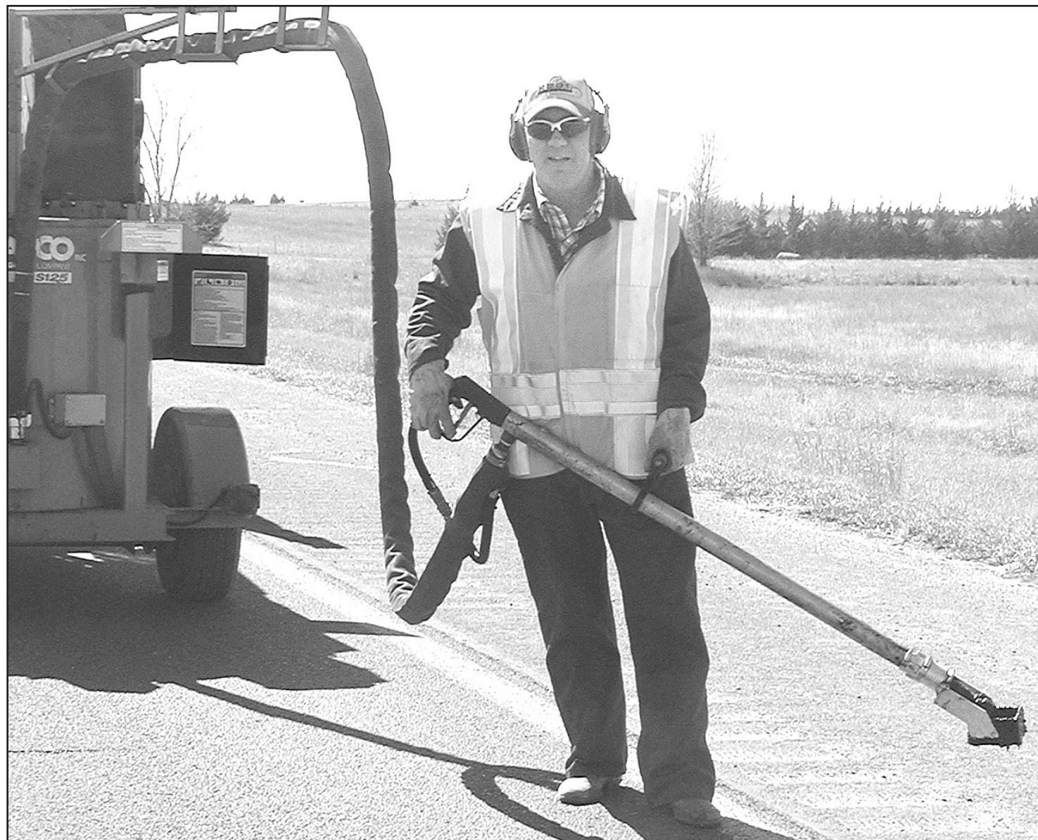
FILLING CRACKS in the pavement just south of Oberlin on U.S. 83, Kansas Department of Transportation workers were busy last Tuesday while the temperatures were in the high 70s. — Herald staff photo by Cynthia Haynes
