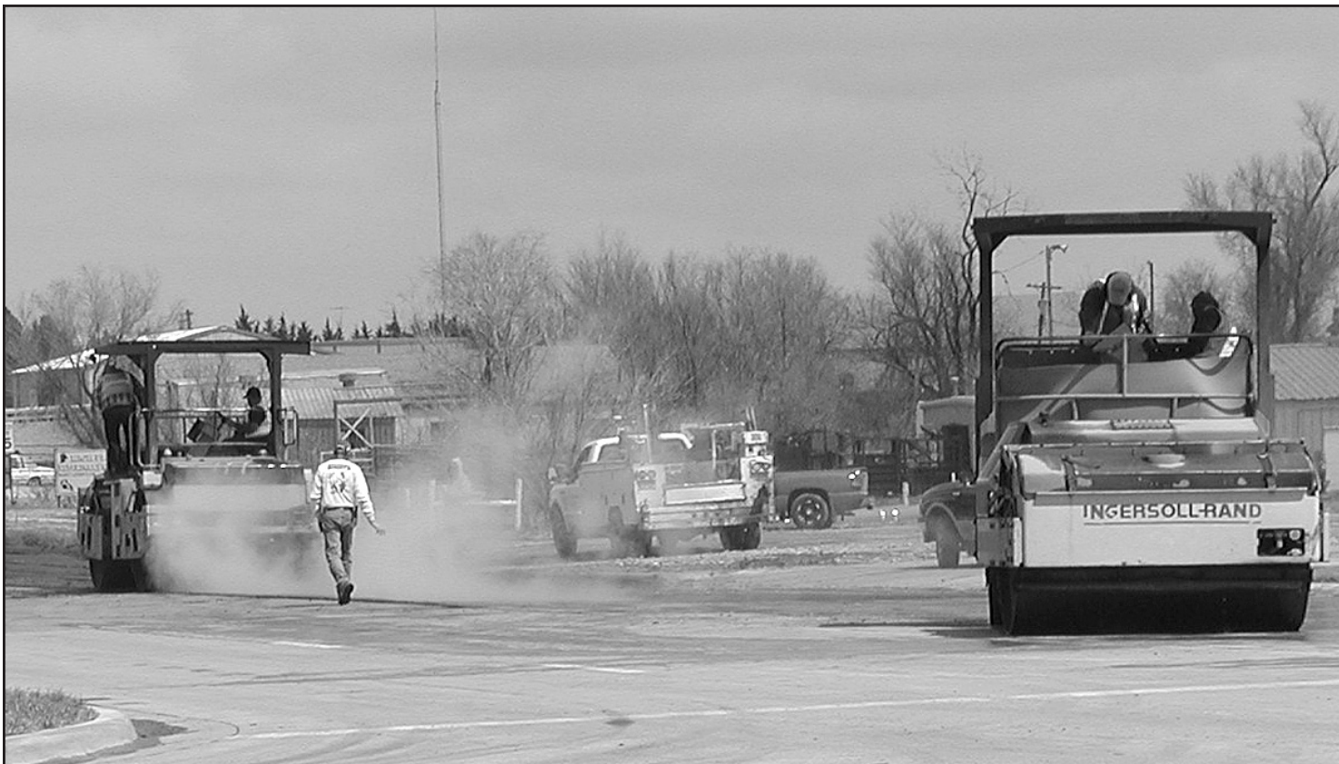
JUST NORTH of the U.S. 36-U.S. 83 intersection, workers with Venture Corp., under a contract with the Kansas Department of Transportation, was putting an overlay on the east side of U.S. 83. — Herald staff photo by Kim Davis
