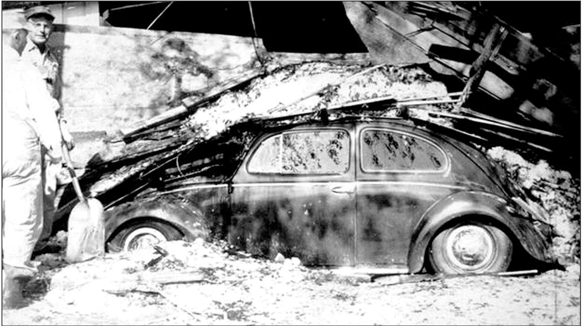
DICK FRIENDLY OF SELDEN drove his Volkswagen under the marquee on the car from the hail's weight. The storm damaged many businesses and of the Farmers State Bank to avoid hail damage, but the marquee collapsed homes, as well as crops.
