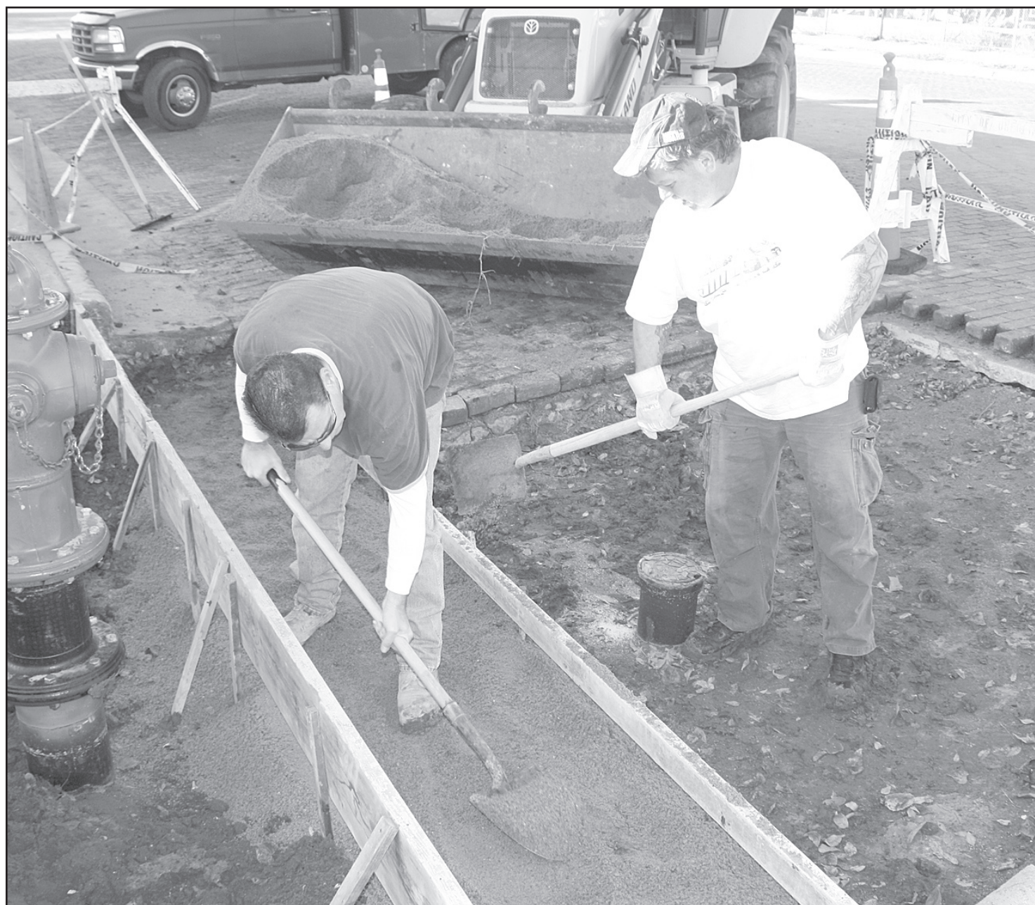
ON THE SOUTH END of Main Street, owner Wayne Hackney and helper Todd Gould from Oberlin Concrete spread sand Monday before they put concrete down. The concrete and bricks needed to be replaced after the city had to fix a water leak near the hydrant to the north of the Last Indian Raid Museum. — Herald staff photo by Kimberly Davis
