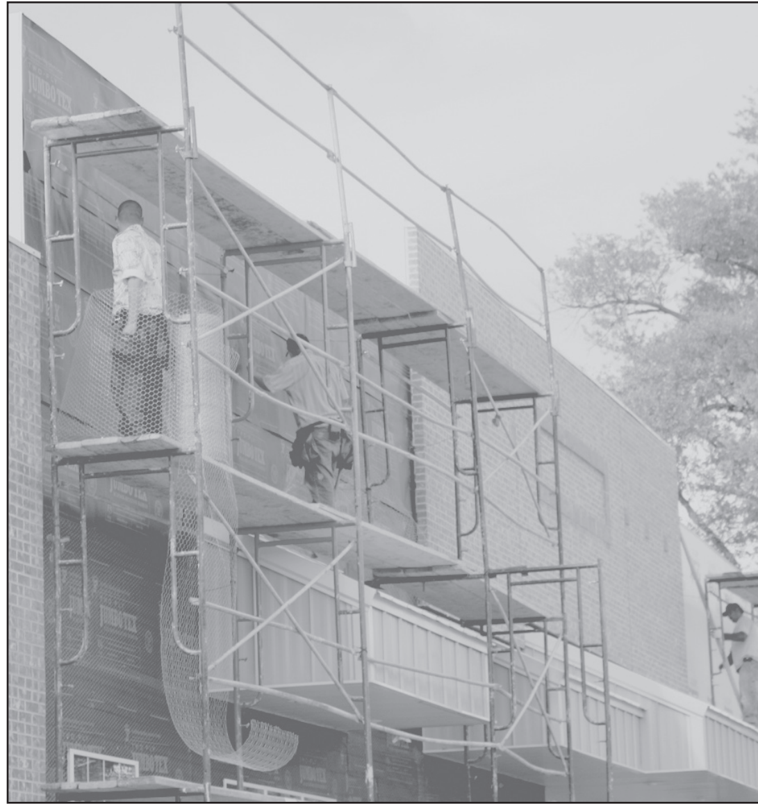
MEN WORKED on the new recreation center in downtown Oberlin on Monday, preparing the front and sides of the building for the first coat of stucco, which will help seal the center from the weather.
