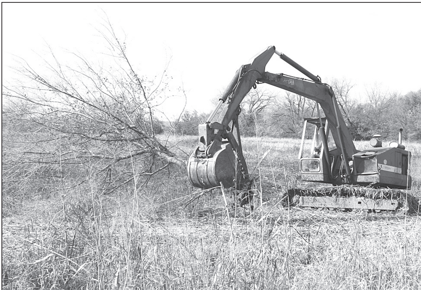
ON MONDAY, contractor Dave Bose was digging out dirt, trees and other plants near the spillway for the wetlands which Pheasants Forever hired him to build in the former
